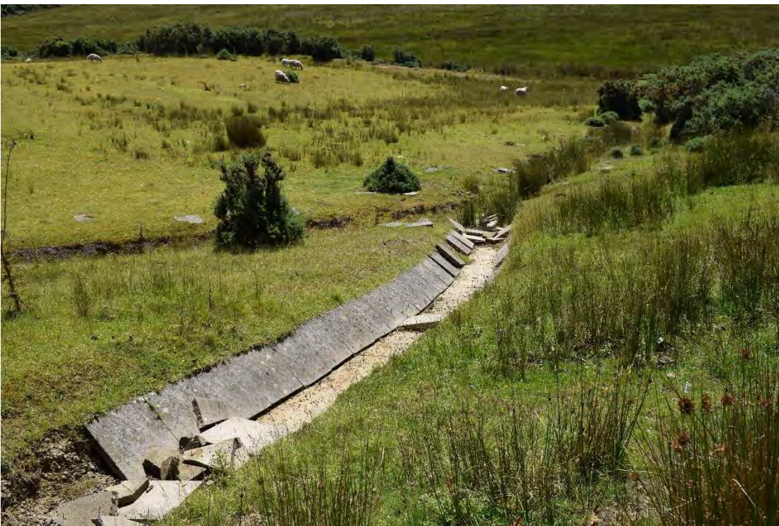
Photo 4: Shows a section of the perimeter drain surrounding the central area of the site.
