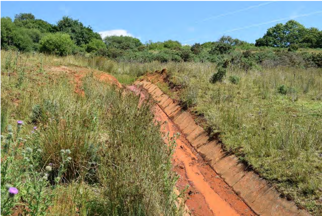
Photo 5: Shows the heavily orange/rust coloured, poorly vegetated drainage channel at the northeast of the site
